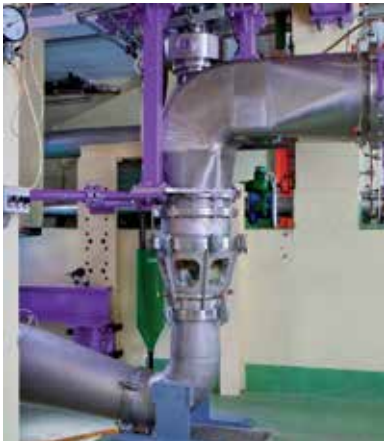
Photo 27. The Diagonal turbine set in Mhylab's test bench.
