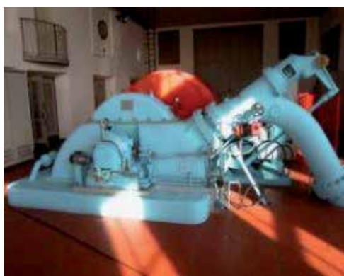
Photo 2. Müllhau: Drinking water turbine (2-nozzle Pelton turbine).
