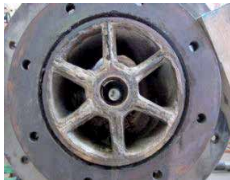
Photo 30. The x-cross liner for a nozzle, worn out by limestone.
