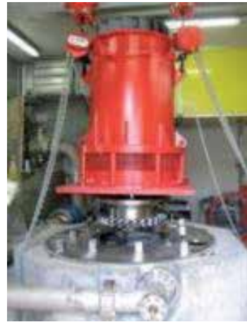
Photo 8. Le Châble Profray: The turbine and its runner and the alternator, during the erection.
