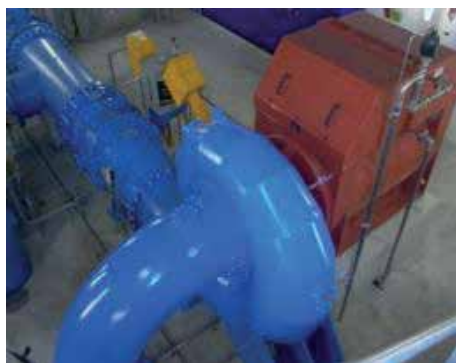
Photo 18. Aire-La-Ville: the Francis turbine set on the attraction discharge, close to the fish pass entrance.
