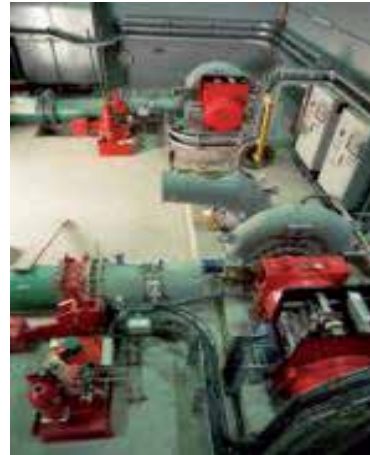
Photo 14. Two Francis turbine set on the treated wastewaters of Amman City, As Samra plants (Jordan) ( H = 42 m, Q = 2 \times 2.3 m 3 /s, P = 2 \times 807 kW, E = 8.6 GWh/year, 2007).
