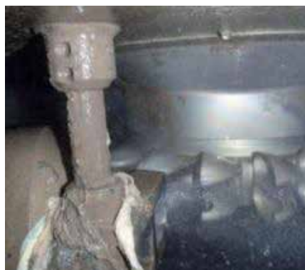
Photo 38. A deflector in the raw wastewater (case study le Châble Profray).
