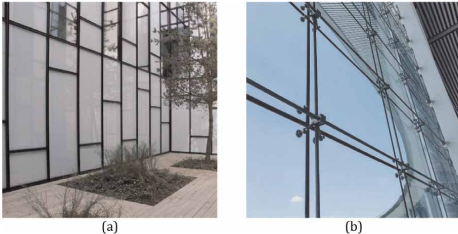
Figure 1. Examples of glass façade; (a) framed glass façade, and (b) frameless glass façade.
