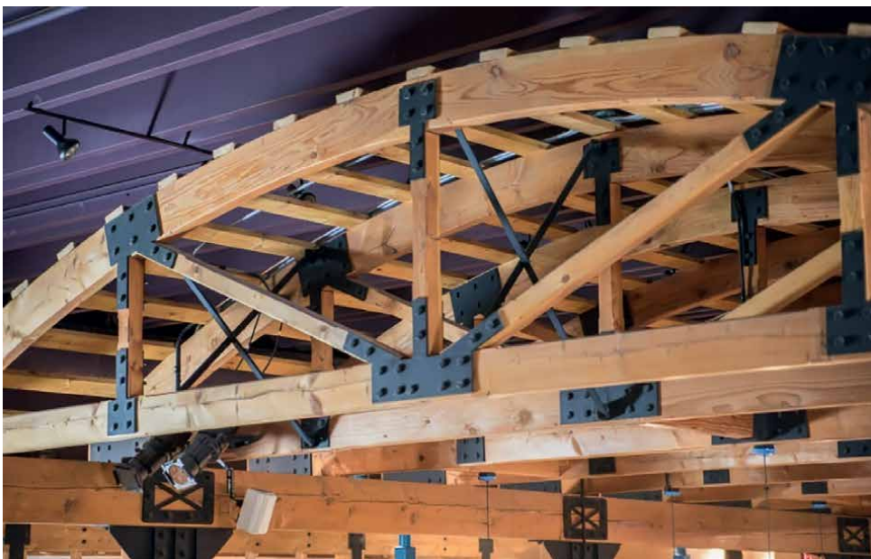
Figure 14. The metallic braces or brackets are used to strengthen the roof structure.
