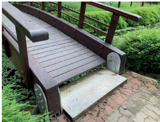
Figure 18. The close-up view of the joinery between the bridge and the foundation using metal.
