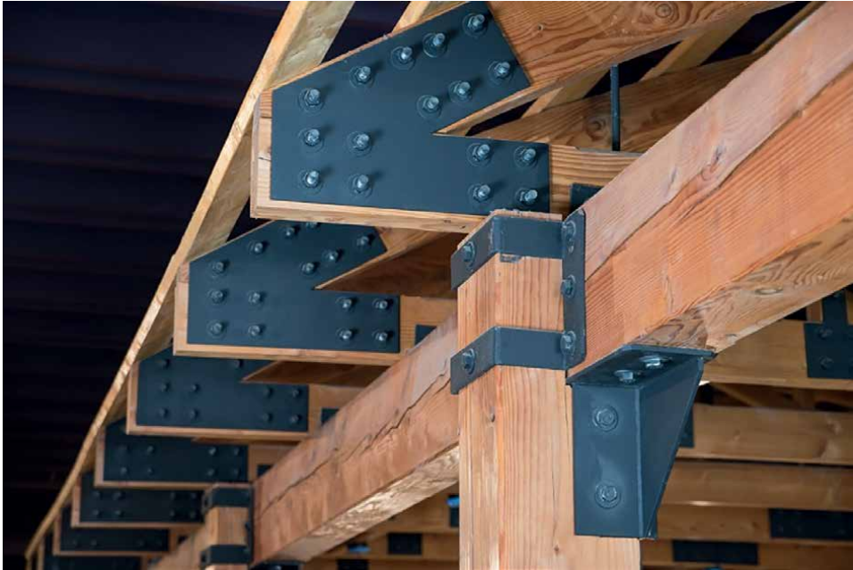
Figure 13. Metallic brackets are used to strengthened the structure between the house beams and poles.
