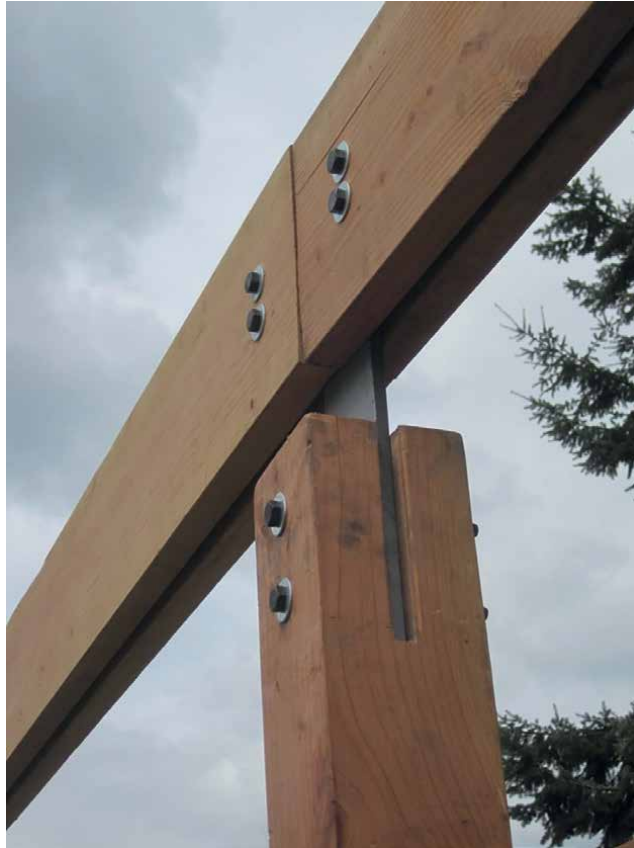
Figure 12. The T-metallic braces used between the laminated timber beam and the pole.
