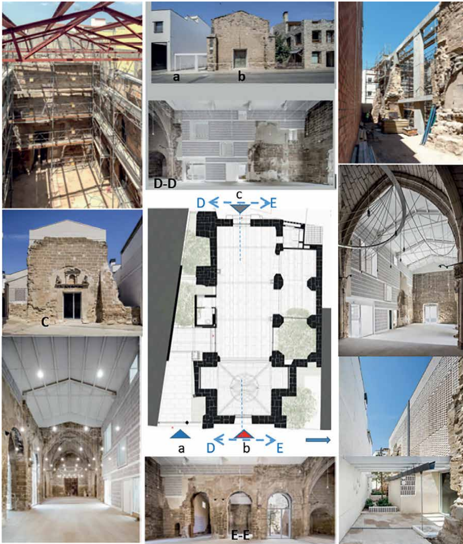
Figure 4. Santa Maria Church of Vilanova: (a) The new eastern entrance, (b) The wooden door in the eastern façade after the intervention, (c) The west façade after the intervention, (D-D) View of the interior wall after the intervention, (E-E) View of the interior arches in contrast to the intervention. The rest of photos are for lighting, materials, and roof during and after the intervention. Source: [33, 34].
