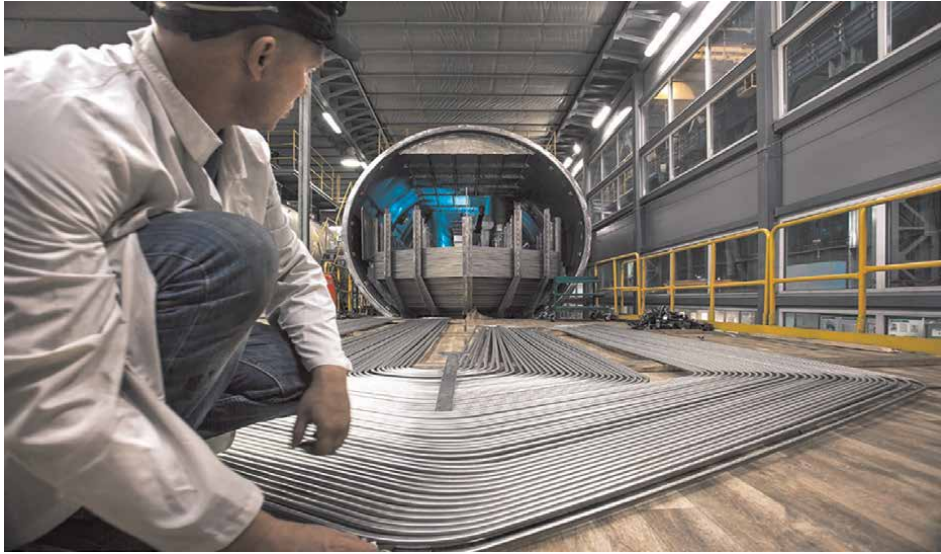
Figure 18. Heat-transfer tubes are installed into steam generator (SG) of PWR (1110 MW el and 3060 MW th ) (in total four SGs per one reactor) (courtesy of Rosatom): https://www.flickr.com/photos/rosatom/36999718643/in/album-72157675727427445/ [Accessed: December 10, 2023]; Photo by E. Lyadov, Atommas, 2016.
