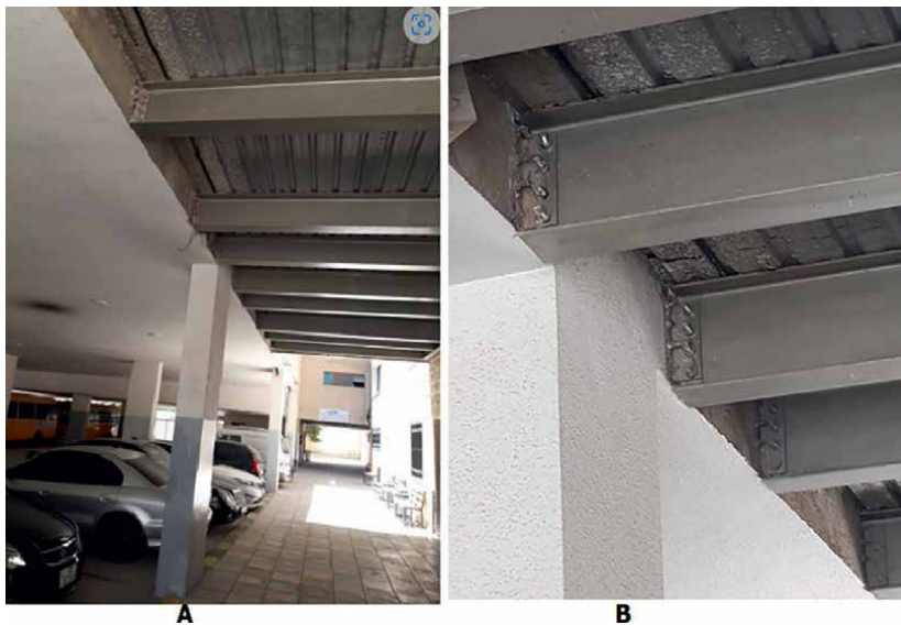
Figure 7. A. Car park building connected to a nearby college building. B. Apparent details of the connection.
