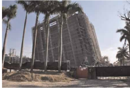
Figure 2. Tilting failure of a new building [3] after the Meinong earthquake in 2016 (Tainan, Taiwan).
