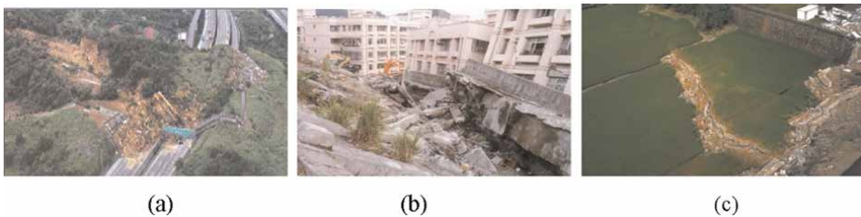
Figure 3. Failure of retaining walls under different conditions [4]: (a) during no rain and no earthquake (Formosa expressway 3.1 K, Keelung, Taiwan); (b) during the rainy season (Lincoln County in New Taipei City, Taiwan); (c) during an earthquake (Quanjiafu Community in Taichung, Taiwan).
