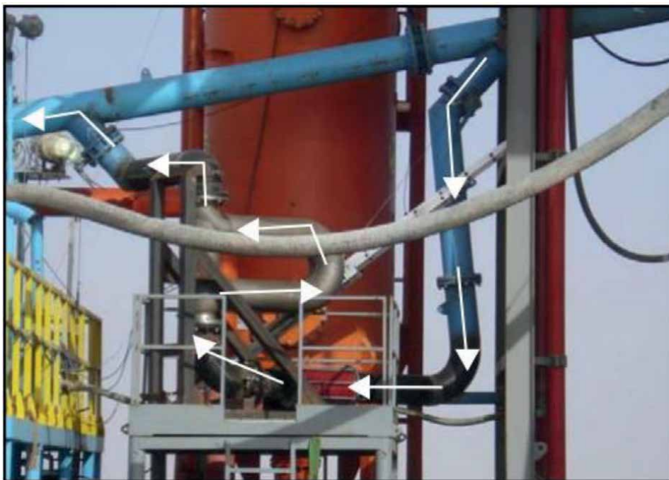
Figure 2. Coriolis installation on the bell nipple of a conventional drilling rig. N.B.: The arrows indicate the bypass and flow direction through the Coriolis from bottom to top [26].
