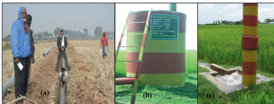
Figure 7. Buried pipeline system: (a) pipe laying stage, (b) header tank for raising pressure head, and (c) outlet with air vent (source: [22]).
