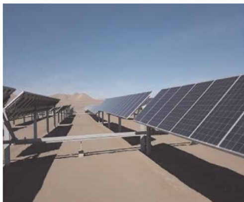
Figure 17. Solar photovoltaic plant Uribe Solar Station near the city of Antofagasta.
