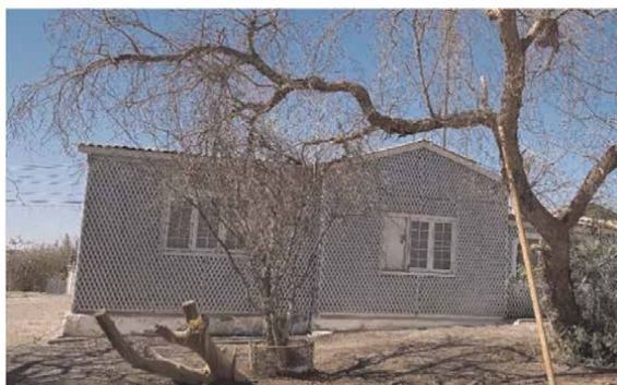
Figure 21. Case of a Chalet house in the María Elena saltpeter office, with a ventilated façade with wooden trellised treillage so that the vine or climbing vegetation covers the architectural envelope.
