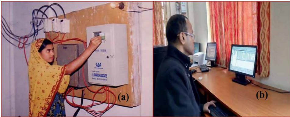
Figure 9. Prepaid metering system: (a) a woman inserts her prepaid card into the irrigation equipment's prepaid meter, and (b) the system is monitored over the internet network from the BMDA's headquarters (source: [22]).
