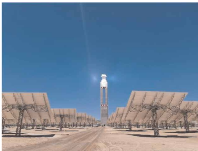
Figure 1. Cerro Dominador: The first Concentrated Solar Power Plant in Latin America with 10,600 mirrors (heliostats) of 140 m 2 each and more than 1,000 hectares, it is capable of avoiding the emission of about 640,000 tons of CO 2 per year and supplying a city of approximately 380,000 homes, located near the saltpeter office of Maria Elena in the Atacama Desert, Chile.
