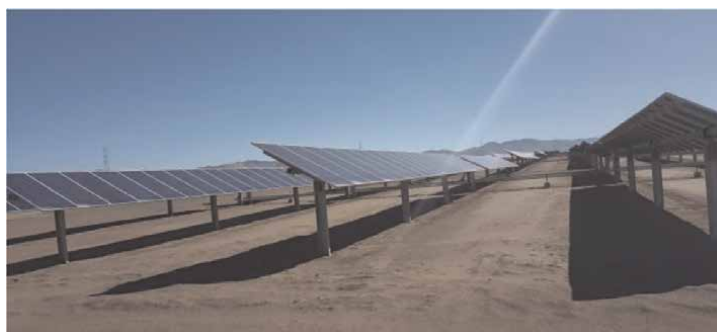
Figure 18. The solar photovoltaic plant designed has a maximum power of 56,632,400 Wp consisting of 182,960 solar modules of 315 Wp, 336 solar trackers on an east-west axis.
