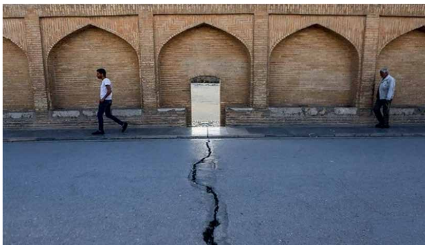
Figure 4. Cracks in thirty-three bridges. Source: [4, 20].
