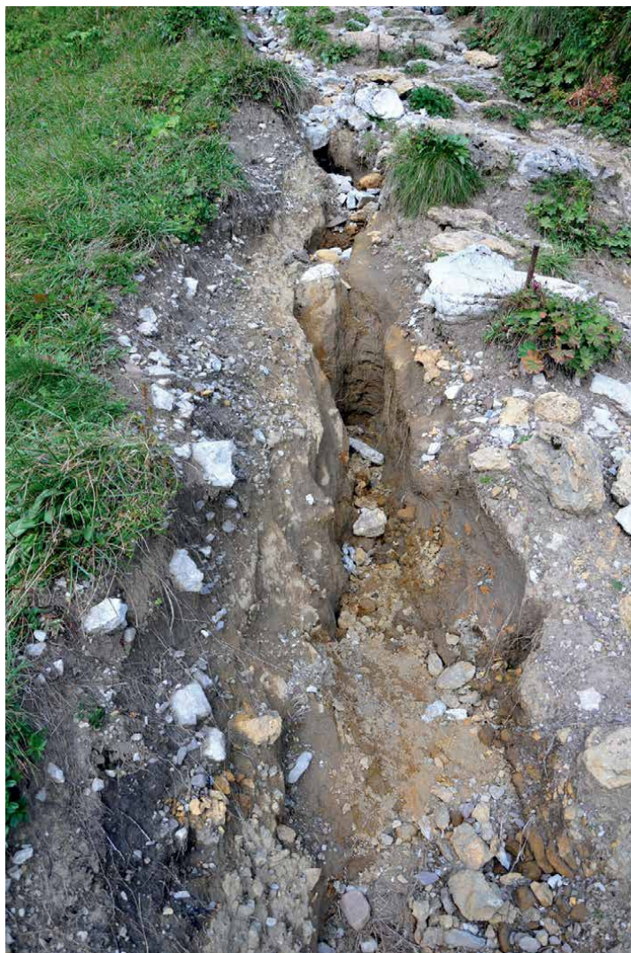
Figure 22. Intensive deep erosion of the hiking trail under Kopské sedlo after an intense downpour in June 2016 (Hreško, 14 September 2016).
