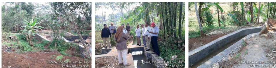
Figure 10. Kreon weir, irrigation network, and irrigated rice fields in Bangunsari Village, Pageruyung District.
