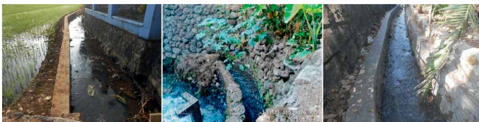
Figure 8. Semi-technical tertiary irrigation channels in Bebengan Village and Ngabean Village, Boja District.
