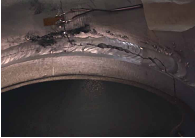
Figure 10. Typical final failure of hand-hole details.
