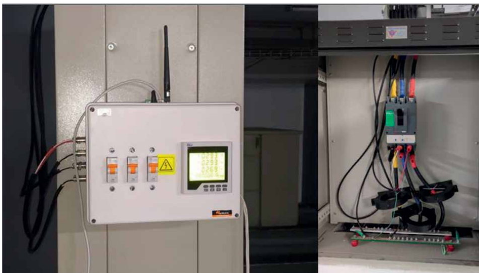
Figure 2. Physical and functional design of the IoT sensor in a distribution board. Source: prepared by the authors.
