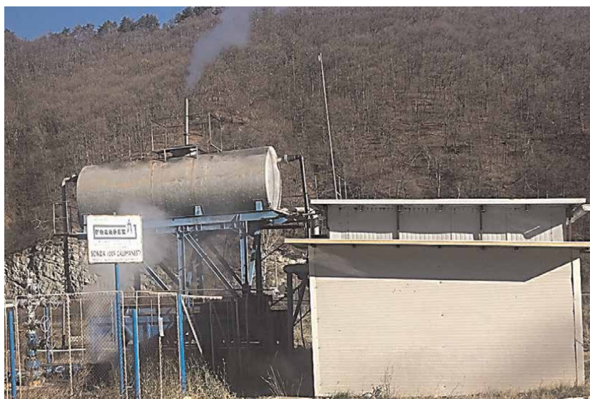
Figure 3. The borehole 1009 and geothermal station (source: photo of the authors).
