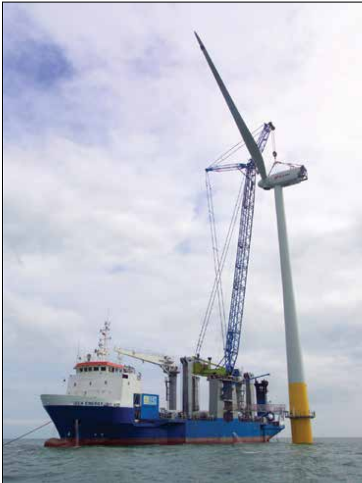
Fig. 22. Wind Turbine being erected with a crane from a special ship at Kentish Flats Offshore Wind Farm, UK (Courtesy: Elsam)
