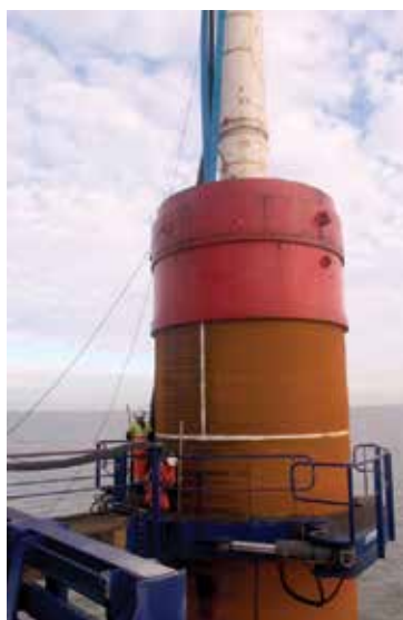
Fig. 8. Menck Pile driving hammer atop a steel pipe pile at Kentish Flats Offshore Wind Farm, UK (Courtesy: Elsam)
