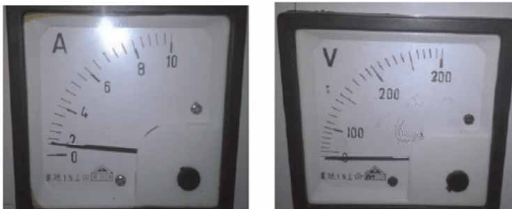
Figure 9. Ammeter and voltmeter.
