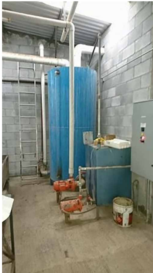
Figure 10. Nitrogen recycling as refrigerant and automation panel.
