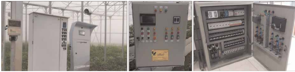
Figure 6. Automation and control of greenhouse using PLC.
