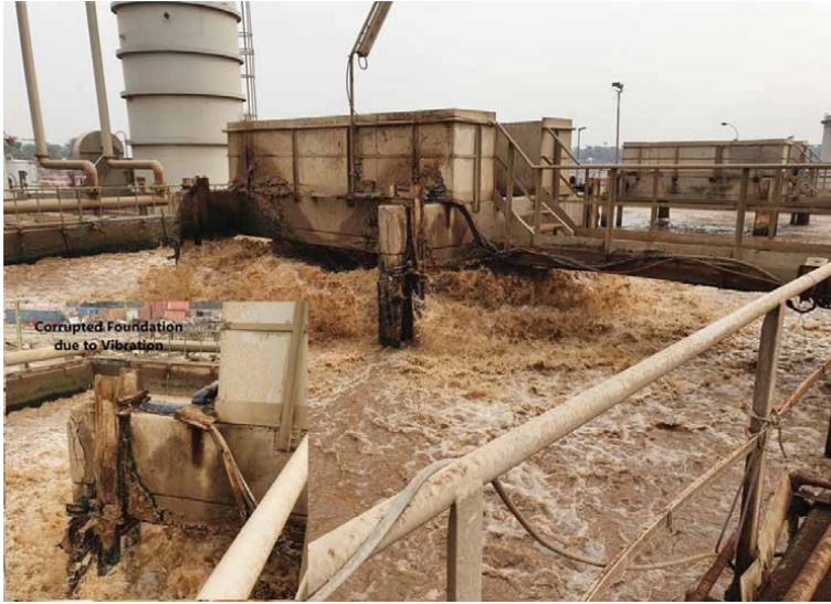
Figure 4. Surface with corrupted foundation due to the vibration.
