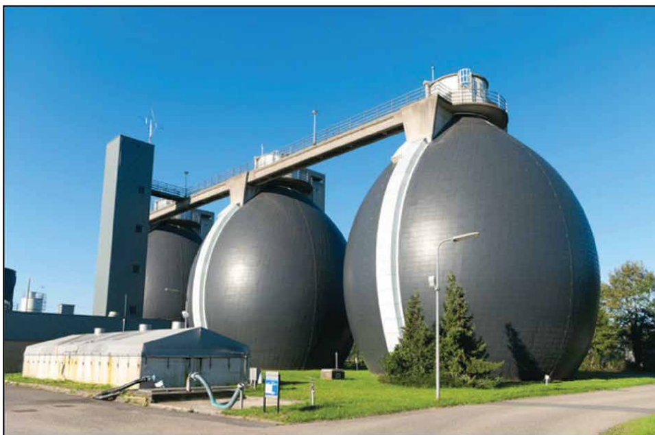
Figure 14. Sewage treatment plant for gas production.
