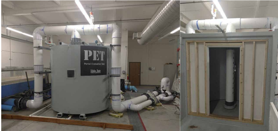
Figure 2. PET tank and piping.
