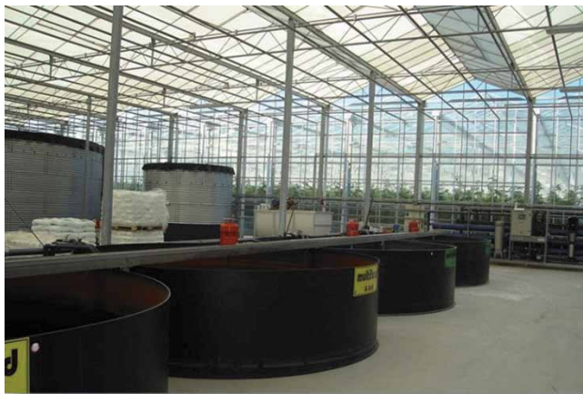
Figure 14. Tanks for water, nutrient solution, and nitric acid used for adjusting the nutrient solution pH.
