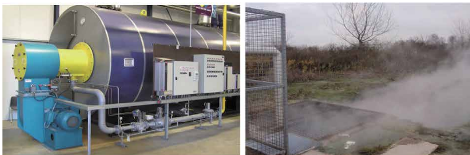
Figure 8. A boiler in the greenhouse boiler room (the Netherlands).
