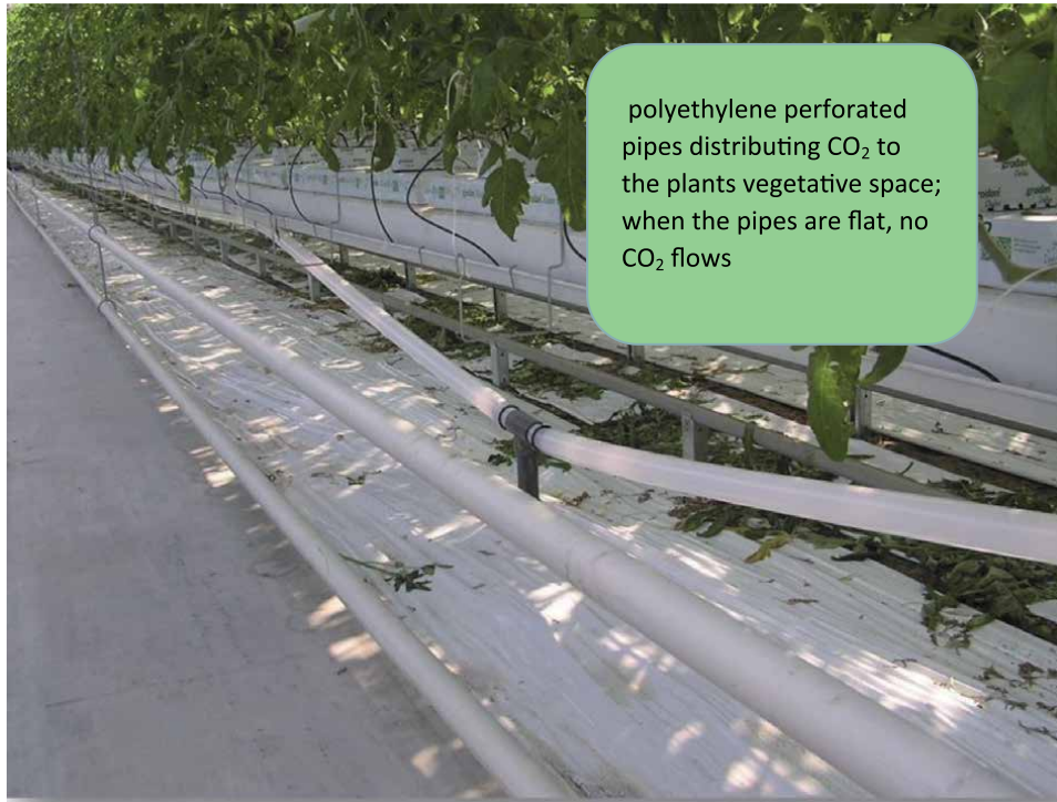
Figure 21. Plastic perforated pipes distributing CO 2 (The Netherlands).
