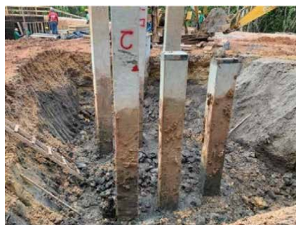
Figure 12. Reinforced piled embankment built for crossing the watercourse in the city of Abaetetetuba, Pará state. a) Stratigraphic profile; b) arrangement of the piles and the geogrid reinforcement, in cross-section; c) installation of piles in the abutment bridge (photo: NS Campelo).
