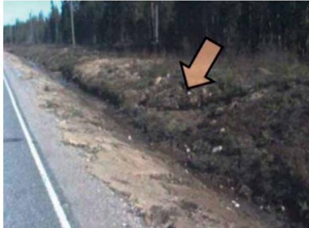
Figure 4. Unstable raceway slope fills the bottom of the channel and causes an annual increment in road surface settlement.
