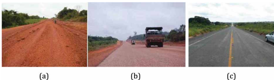
Figure 7. Use of SCACC in highway paving: a) scattering of the mixture of lateritic soil and SCACC for the execution of the base course; b) completed experimental runway, with asphalt course in double surface treatment. c) Conditions of the experimental runway approximately 2 years after completion [4].
