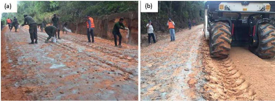
Figure 2. a) Distribution of cement and ZS additive in the experimental runway by manual spreading; b) homogenization of the soil, cement, and ZS additive in situ by means of a recycler [1].
