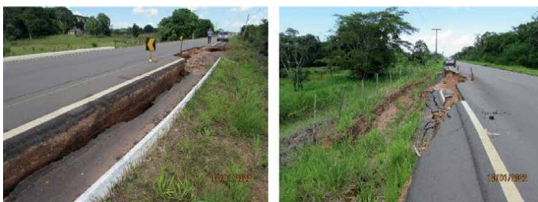
Figure 23. Rupture of road slopes, after the river ebb cycle (photos: NS Campelo).
