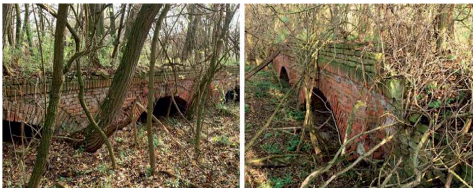
Figure 11. A view of the bridge at the time of project preparation before the renovation.
