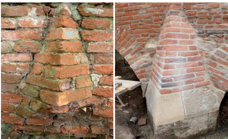
Figure 8. A detail of the original edge of the bridge column. A detail of the edge of the bridge column after the repair.
