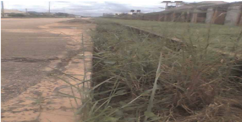
Figure 1. A waterlogged open concrete drain overgrown with weeds in new Owerri Nigeria.
