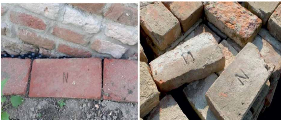
Figure 9. Baroque bricks taken out of the loosened structures of the bridge were reused in its restoration. They are marked with the letter N (Nicolsburg).
