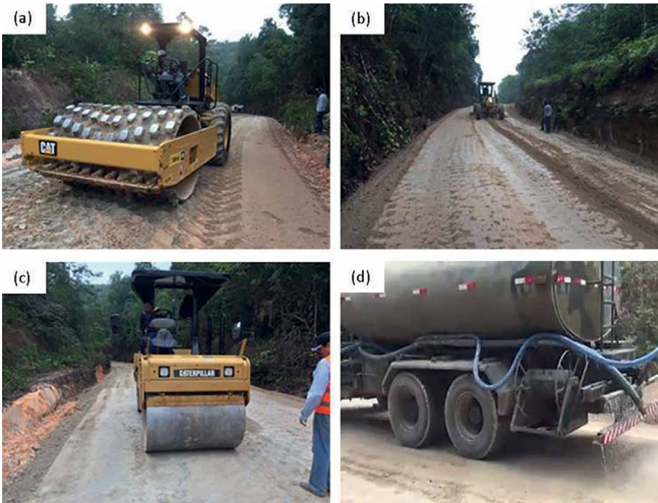
Figure 3. Steps of a) compaction; b) bulging; c) surface finishing; and d) curing of the stabilized base [1].
