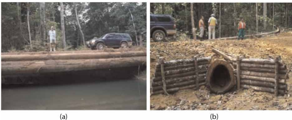
Figure 20. Use of wood in the drainage of igarapés crossing roads with low traffic volume in the Brazilian Amazonia. (a) Wooden bridge ( pinguela ); (b) hollow wood “tube” [110].
