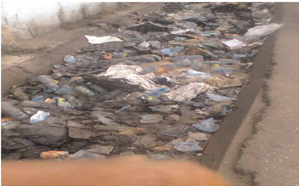
Figure 2. A waterlogged open concrete drain being used as a waste dump site in new Owerri Nigeria.
