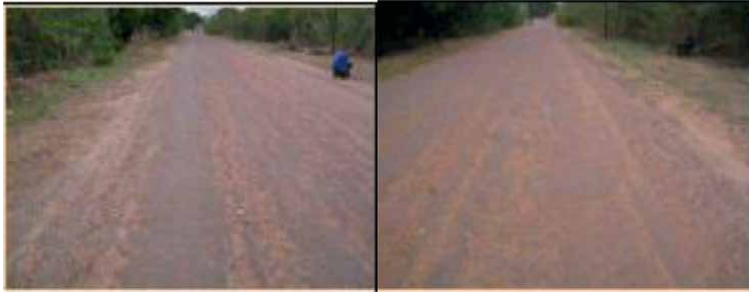
Figure 10. Surface condition of the stabilized base with asphalt emulsion after 20 months of execution [5].
