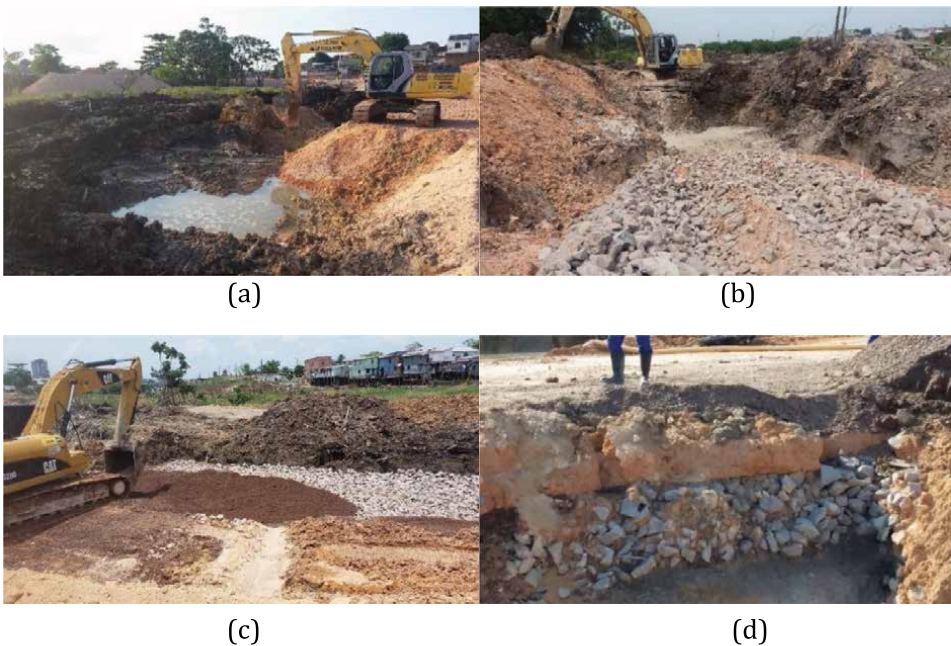
Figure 18. Construction of an urban corridor with partial replacement of the natural ground with low bearing capacity. a) Partial excavation of the layer; b) placement of the coarse crushed stone material ( rachão ); c) placement of the embankment layer for road construction; d) appearance of the rachão layer after partial implementation of the compacted earthen embankment (photos: NS Campelo).
