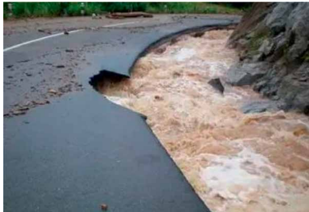
Figure 5. Road channel fracture due to lack of proper slope angle.
