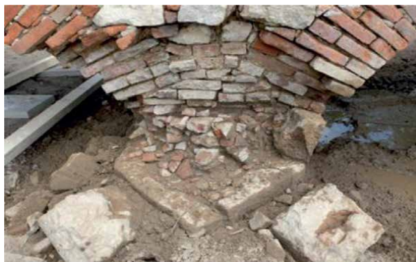
Figure 7. To determine the foundation of the bridge, it was necessary to carry out a borehole probes.
