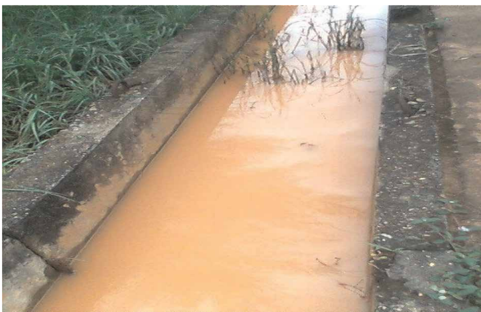
Figure 4. A stagnant pool of water in an open concrete drain in new Owerri Nigeria.
