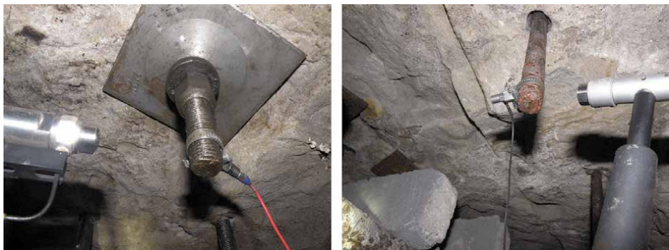
Figure 9. Impact excitation of installed rock bolts, with the working prototype (left) and the unit fulfilling ATEX requirements (right).
