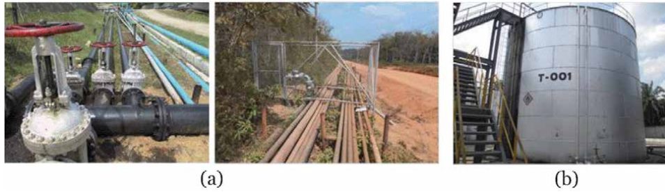
Figure 1. Pipeline system and storage tank for oil gathering activity. (a) Pipeline System. (b) Storage Tank.
