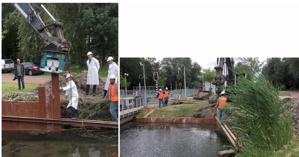
Figure 11. Installation of retaining wall by vibrating profiles with EoL composite in the soil [3].
