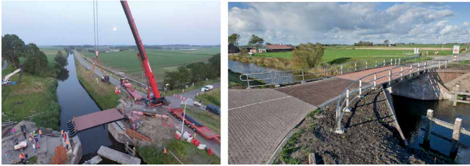
Figure 15. Dinzer bridge with deck profiles of re-used composite: Installation and final result [15].
