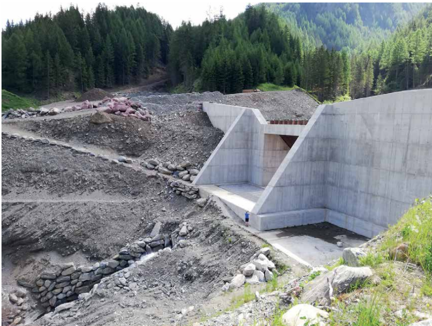
Figure 7. Technical measure against debris flows upstream of the buildings in Figure 6 . The site was visited during a GreenRisk4Alps field trip in June, 2019 (source: © S. Cocuccioni).
