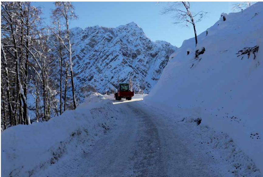
Figure 16. The Macesnovec-Drnice forest road enabled access to the construction site (photo: Jurij Beguš).
