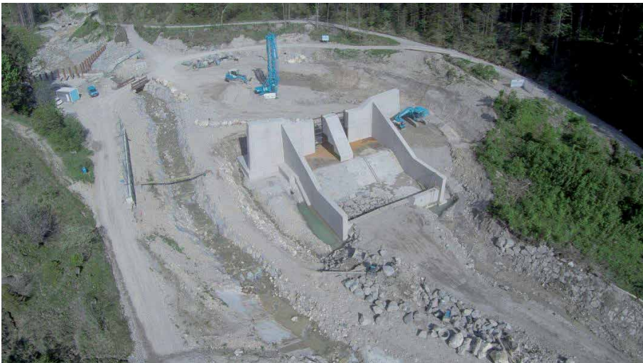
Figure 9. View of the completed barrier structure. A driftwood rake can be seen in the background on the left [12].
