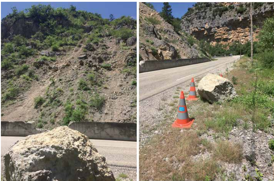
Figure 4. Example of rockfall risks in the park (photos F. Berger INRAE).
