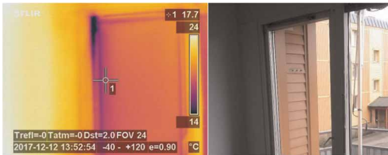
Figure 4. IR-thermography picture showing thermal bridges around the window in Centralgatan 14.
