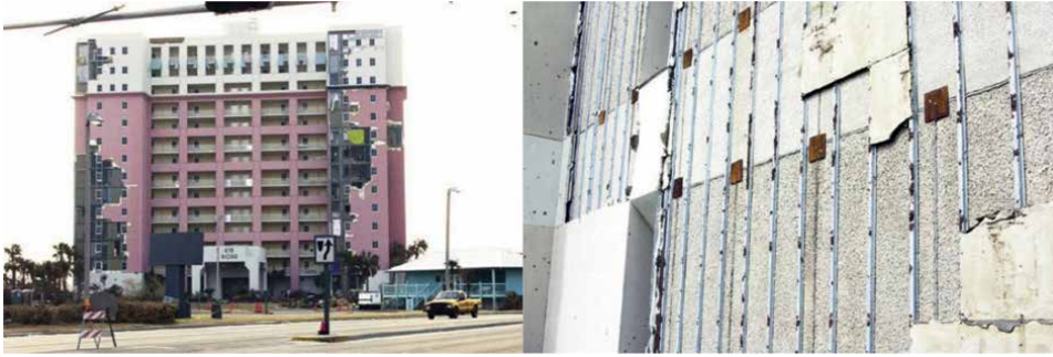
Figure 8. Detachment of the plasterboard panel from the wall substructure in Pensacola (Florida) [34].
