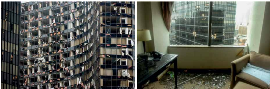
Figure 9. Extensive damage due to wind action and flying debris to the opaque and transparent façade of the Hyatt regency hotel (New Orleans) [8].
