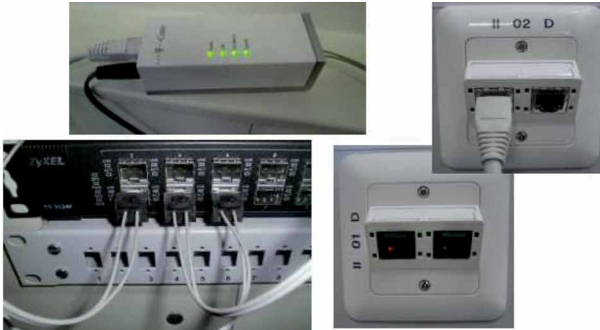
Figure 15. POF media converters, Ethernet switches and 4-port optical POF switch RJ-45 wall outlets with WiFi-Accesspoint (Rutenbeck GmbH).
