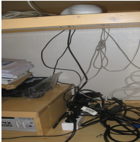
Fig. 1. Cables messing the space under your desk in the office.
