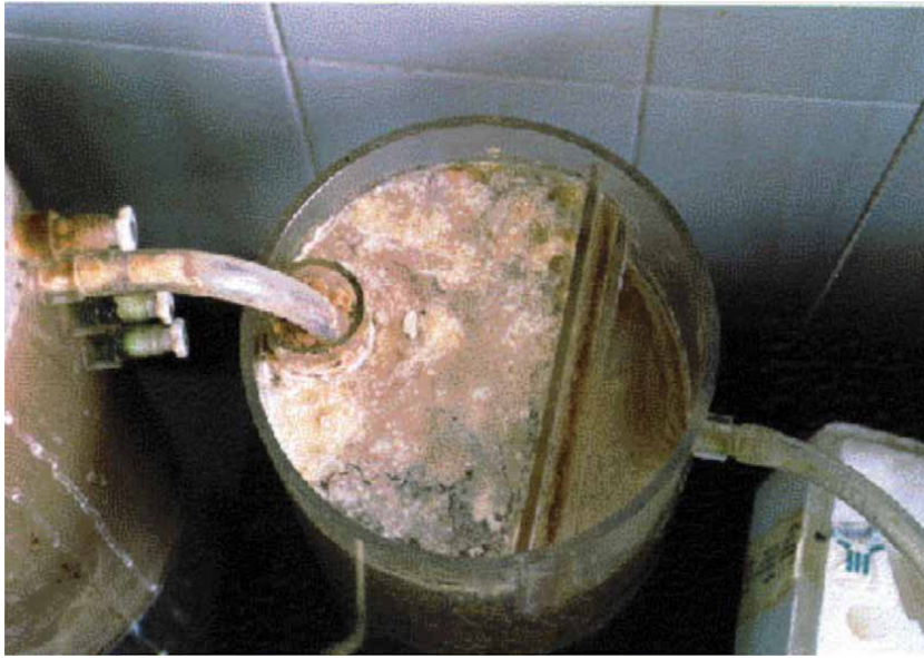
Figure 3. Oil and grease accumulated in settling tank.
