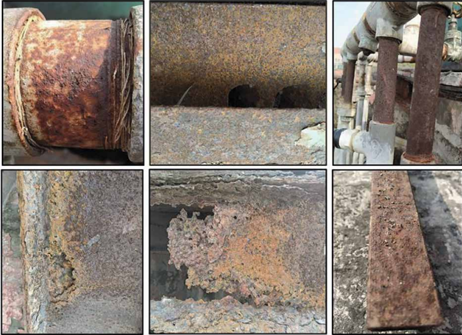
Figure 1. Effect of corrosion on different metallic structures.
