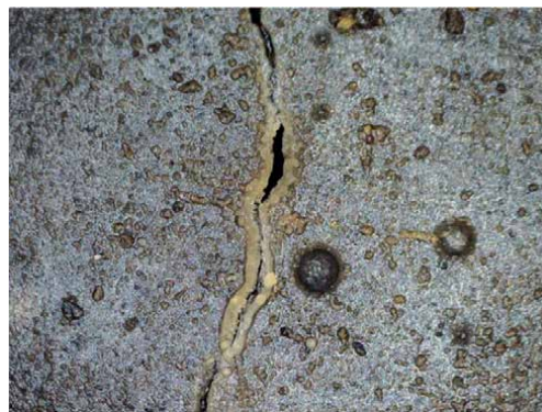
Figure 5. Concrete sample with self-healing process activated [115].
