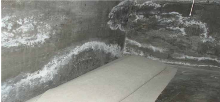
Figure 3. Excessive surface salt due to efflorescence phenomena.
