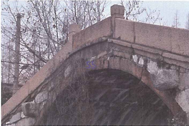
Figure 25. The damage to the slender Yongying bridge.
