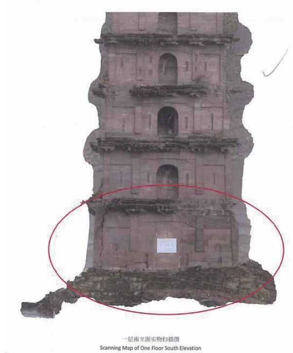
Figure 27. LiDAR scan of the white pagoda surface erosion.
