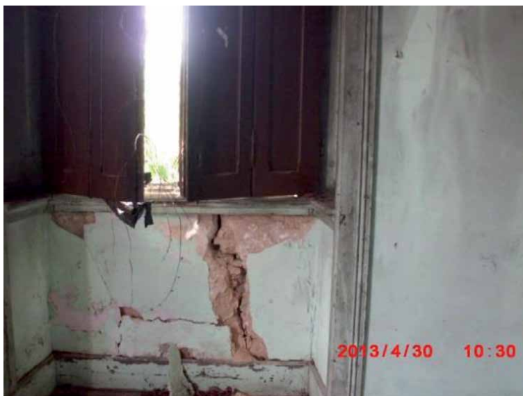
Figure 8. F4 fissure (inside).
