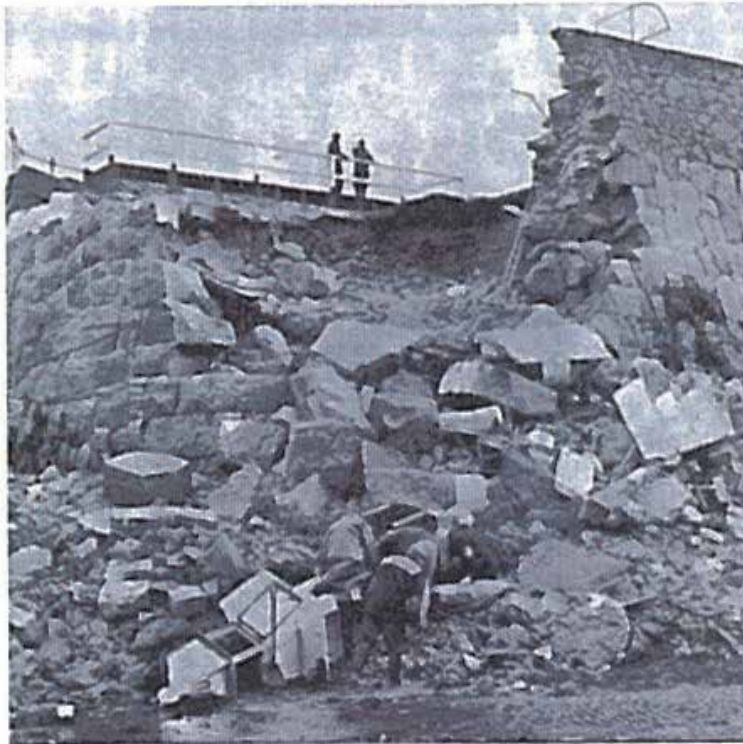
Figure 6. Collapse of Pierhead in 1965 (archives), Ref. [9].
