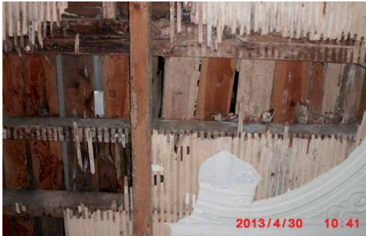
Figure 14. Ceiling under the Sanit. Inst.
