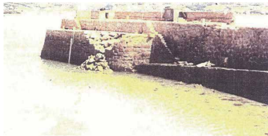
Figure 2. St Aubin's fort breakwater failure 1972 (archives).
