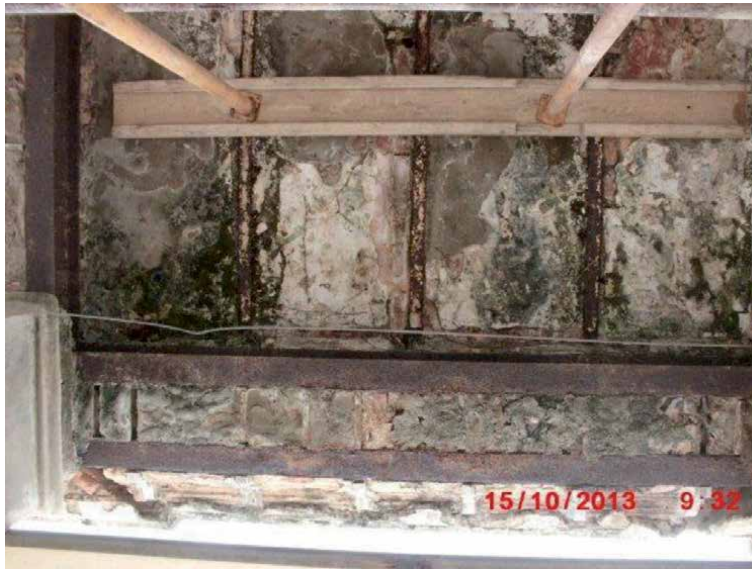
Figure 12. Corrosion of metallic elements.
