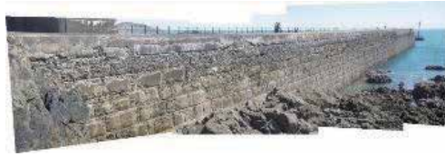
Figure 29. The damaged west side of Elizabeth Castle breakwater.
