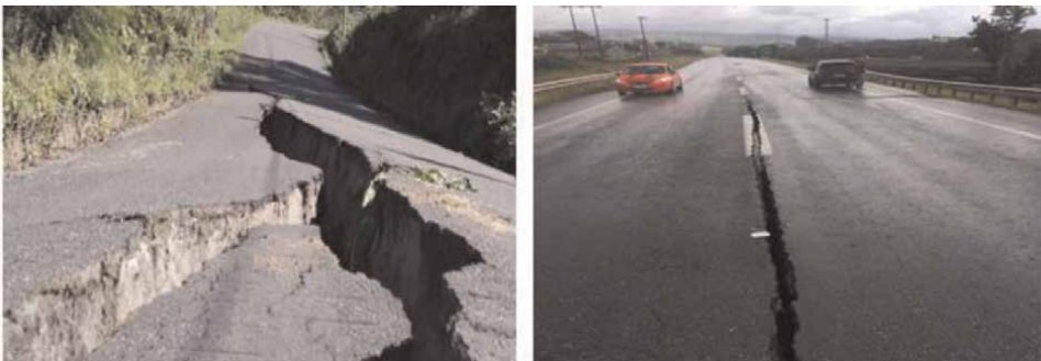
Figure 4. Damage to roads caused by earthquakes, left: Chiapas, 5.6 r earthquake, right: Oaxaca, 5.2 r . Source: Google.
