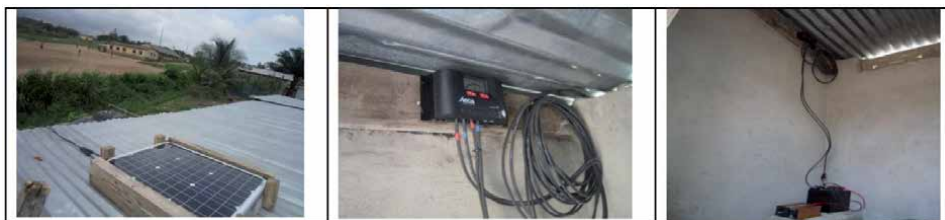
Figure 7. Components of solar-photovoltaic system installed on the biogas digester.
