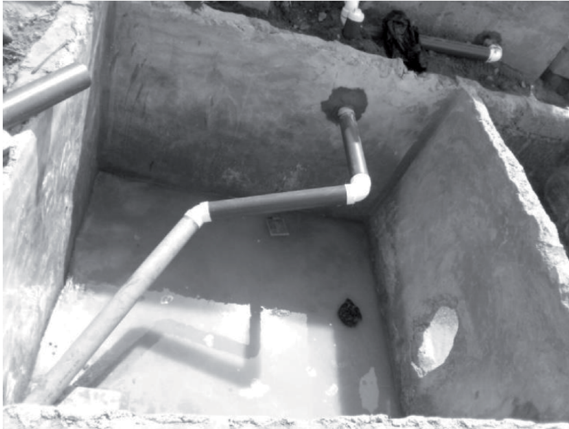
Figure 6. Pipe connections from the pour-flush toilet into the innovative household biogas digester.
