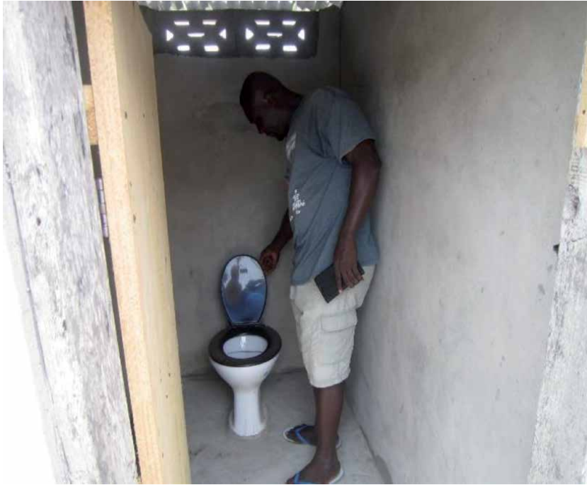
Figure 5. A 3-litre pour-flush toilet seat connected to the biogas digester.
