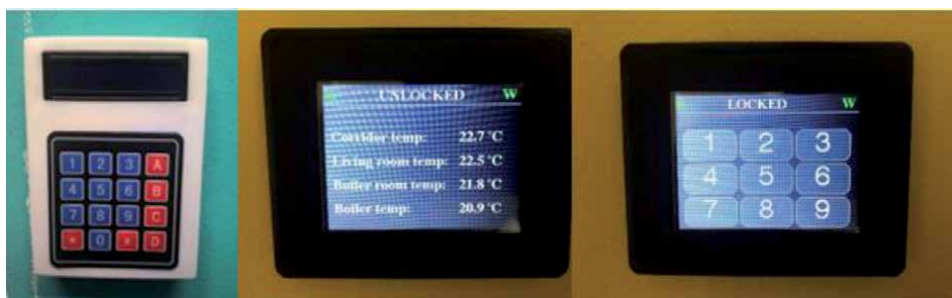
Figure 2. Input board in boiler room.
