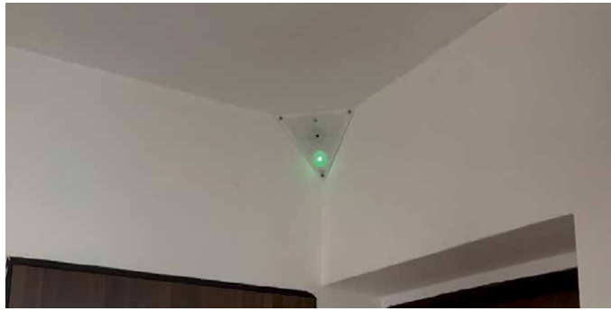
Figure 12. Installation of the ESP32 cam module in the living room.
