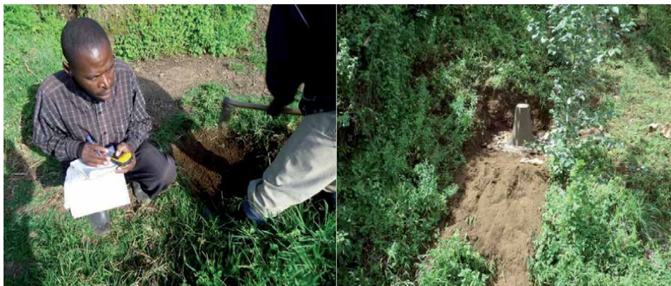
Figure 8. Land demarcation and installation of the benchmarks for land consolidation purpose. Source: GWLM project.
