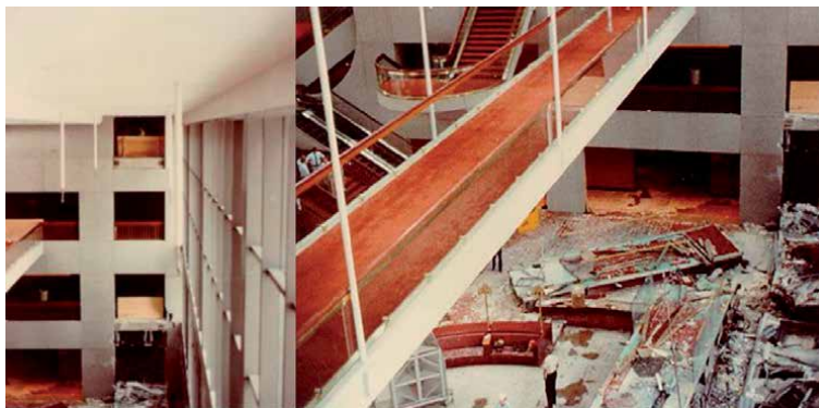
Figure 4. Collapsed skywalk bridge in Hyatt Regency Hotel.
