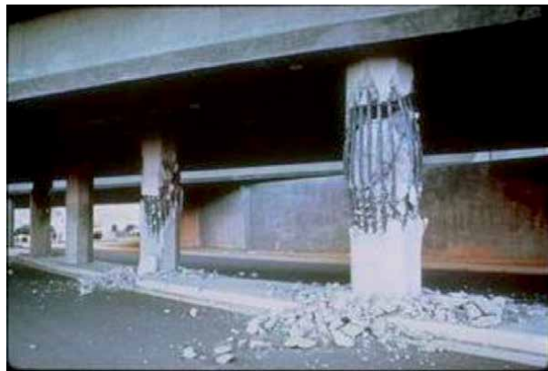
Figure 10. Failed highway bridge columns on Santa Monica Freeway.
