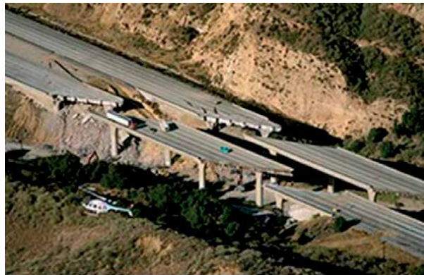
Figure 8. I-5 Newhall bridge failure near SR14.
