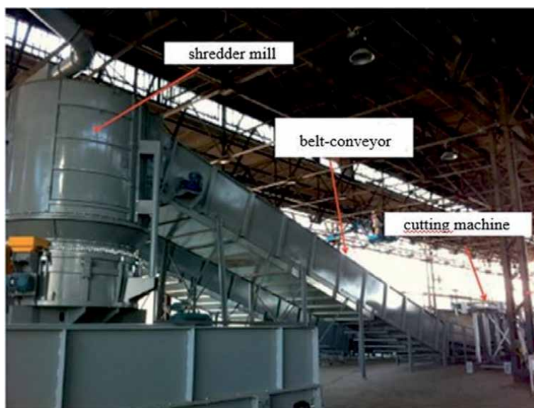
Figure 5. Straw feeding plant: Shredder mill.
