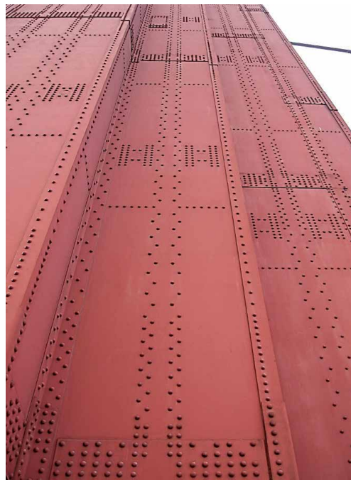
Figure 3. Thousands of rivets are used in the structure of the Golden Gate Bridge, San Francisco, United States.
