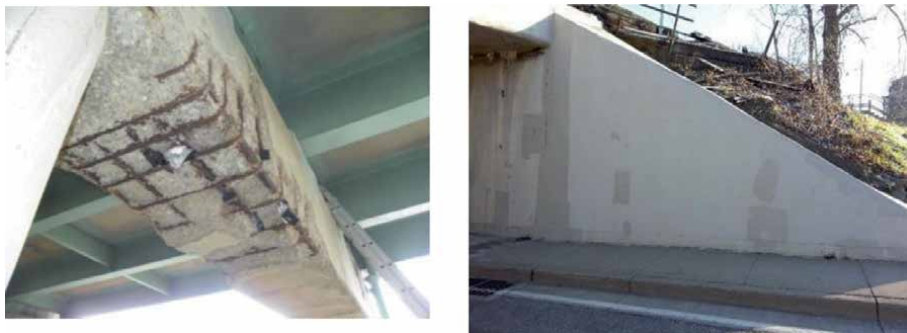
Figure 3. Degradation and retrofitting of highway bridges in West Virginia. (a) Spalling of concrete and exposed rebars of bridge superstructures (courtesy of WVDOT–WVDOH); (b) retrofitting of highway bridge wing walls using GFRP wraps (courtesy of WVDOT–WVDOH).
