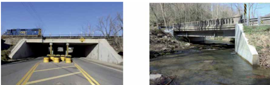
Figure 6. Two bridges in West Virginia Department of Transportation's inventory. (a) East Street Viaduct Bridge (courtesy of WVDOT - WVDOH bridge inspection reports 2012 and 2017); (b) Flag Run Bridge (courtesy of WVDOT - WVDOH bridge inspection reports 2016).
