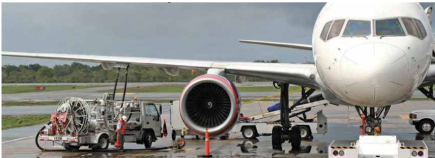
Figure 10. Centralized underground fuel system and hydrant fuel truck.
