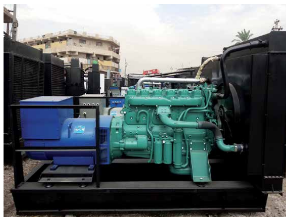
Figure 2. Locally assembled neighbourhood generator (Source: Author).
