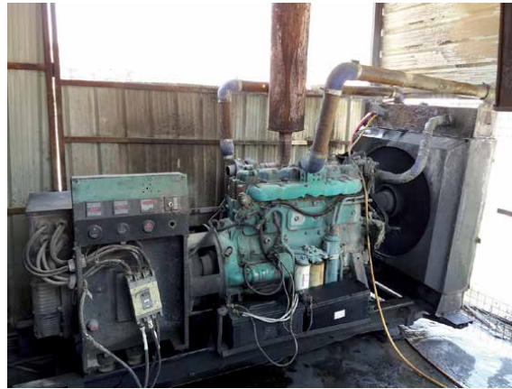
Figure 8. Neighbourhood diesel generator with enclosures removed showing exposed fan (Source: Author).
