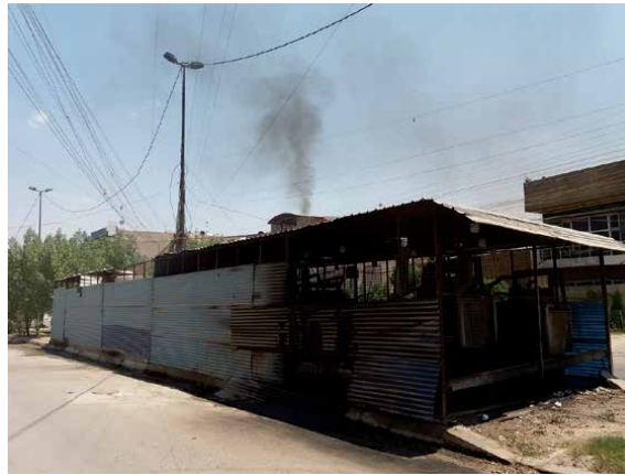
Figure 4. Neighbourhood diesel generator installed on a mid-road pavement in Baghdad (Source: Author).
