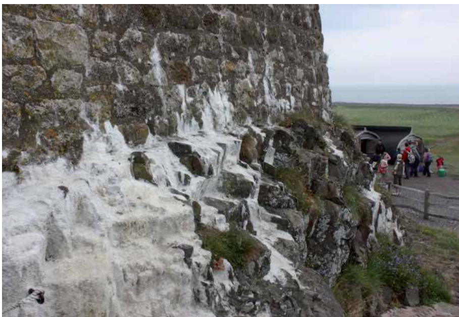
Fig. 1. Speleothem (flowstone) attributed to carbonate leaching from lime rich mortar, Lindisfarne Castle, Northumberland, UK.
