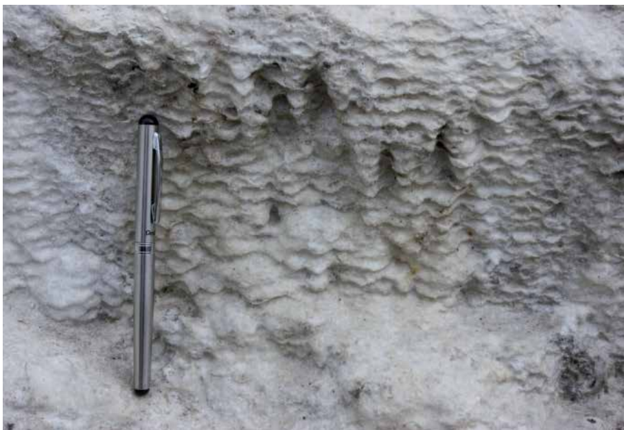
Fig. 2. Speleothem (flowstone) attributed to carbonate leaching from lime rich mortar, Lindisfarne Castle, Northumberland, UK.
