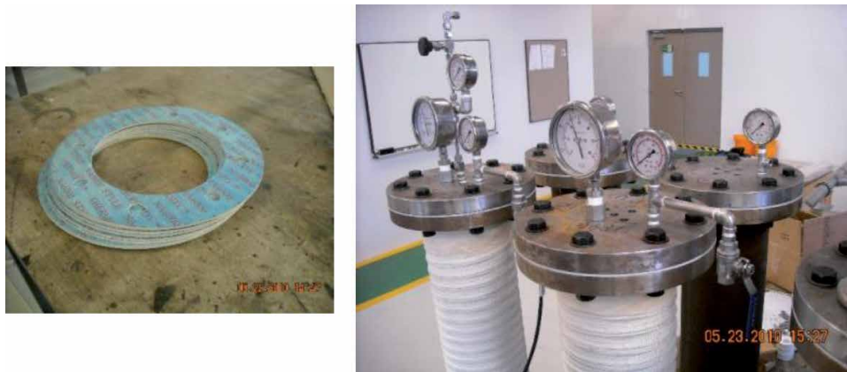
Figure 9. High temperature–pressure gaskets (left); joining of packer and casing flanges, and fixing of pressure and temperature gauges (right).
