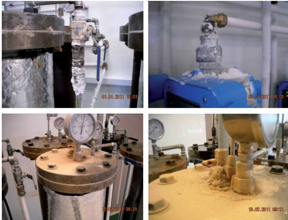
Figure 13. Salt deposition on pipes, fittings, and pump units due to water leakage (top); corrosion of pipes and fasteners due to water leakage and salt deposition (bottom).
