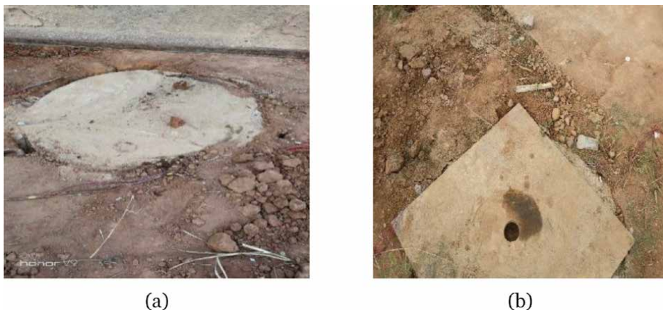
Figure 16. Failure modes of concrete piers. (a) Soil around the pier when the precast pier foundation of recycled compound concrete was destroyed, (b) soil around the piers when the foundation of the cast-in-place ordinary concrete was destroyed.
