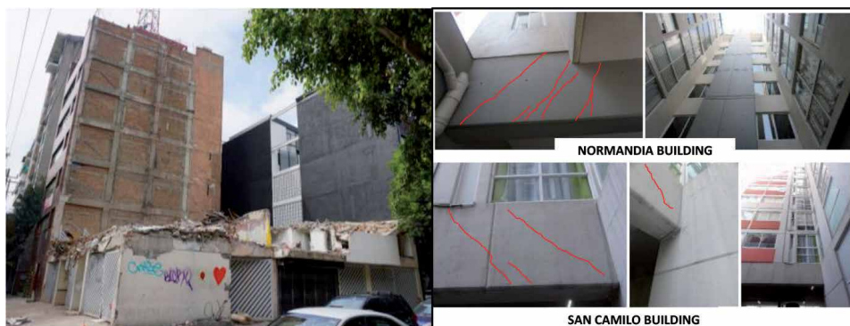
Figure 1. (a) left: Collapse of a building with discontinuities in elevation; (b) right: Diagonal cracks in the girders of the transfer floor in two buildings supporting six and seven stories, respectively.
