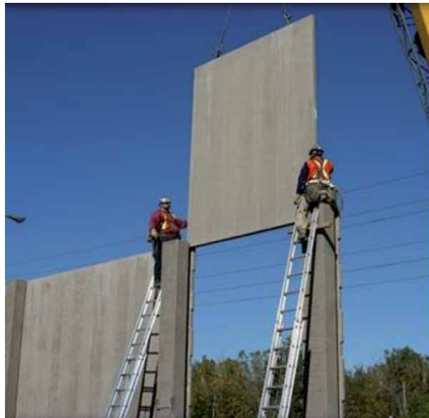
Figure 5. Precast concrete noise barriers.
