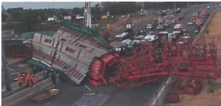
Figure 8. Collapse of temporary supports 2018 (figure reproduced from Ref. [27]).
