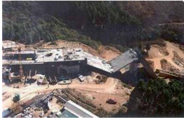
Figure 10. Failure of a multi span bridge (figure reproduced from Ref. [29]).
