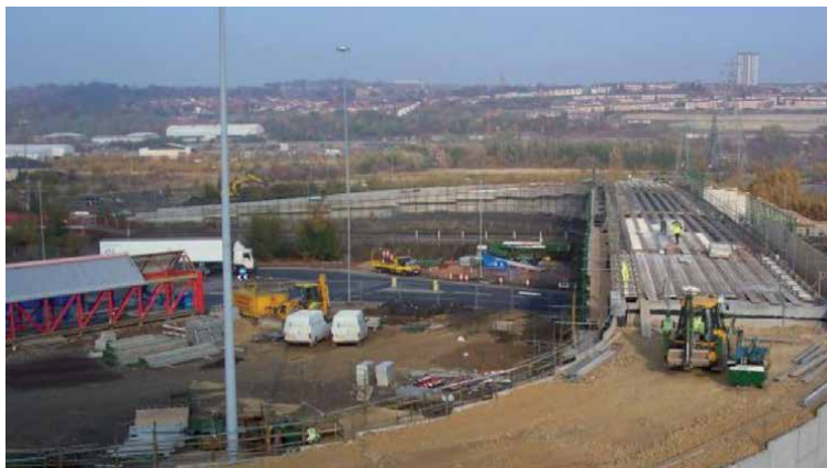
Figure 2. Precast beams and cast in situ deck with GRP panels for formwork over existing highway—4 span bridge.
