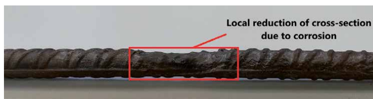
Figure 4. Local reduction of cross-section due to corrosion.
