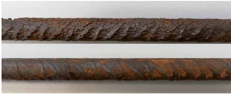
Figure 5. Corrosion damage on steel surface. Inner half of steel bar's circumference (up) - outer half of steel bar's circumference (down).
