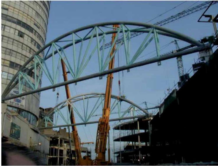
Figure 20. Erection of 140 T truss over the railway with a soil cover of 3 m.
